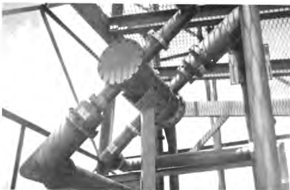
FIG. 9. Candid photograph of the combiner in its mount at the base of the tower. The two 6-inch lines deliver the diplexed power from the transmitters and the 3-inch lines connect to the power-dividing tees shown in the block diagram of Fig. 7.
