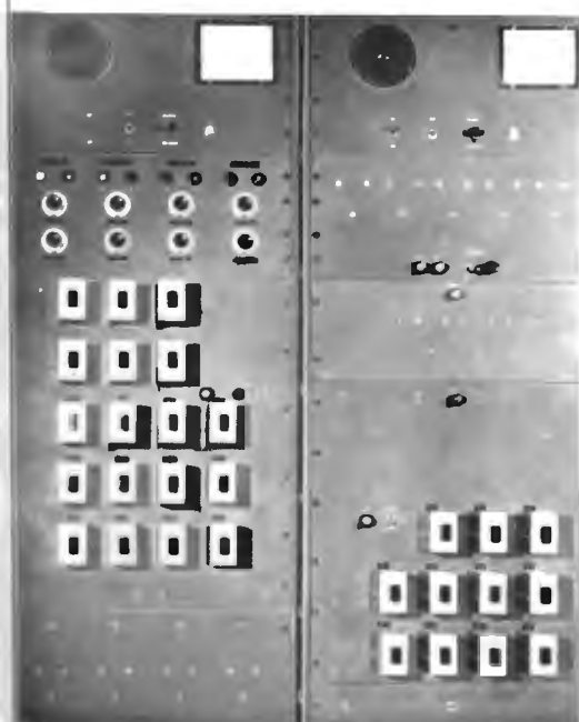
FIG. 8. Close-up of the remote-control racks shown in FIG. 6. At top are the two BTR-20C "slave" units. The remaining equipment in these two racks is custom-built gear for the WBAL remote operation.
