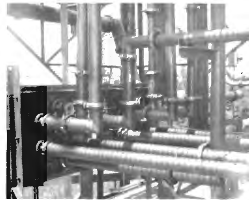
FIG. 19. Snapshot photograph of the manual power-switching complex at the tower base. Shown at left are the switch panels with the (Universal) transmission-line connections.
