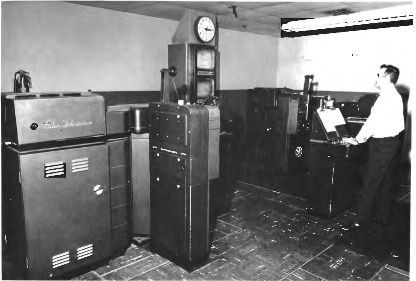
FIG. 19. Film Projection Room. Equipments are operated by the projectionist-switcher at an RCA custom-built control pedestal. They may also be remotely controlled from Control "A" or Master Control. One monitor is for "off the air" viewing, the other is switched from the control pedestal for previewing.
