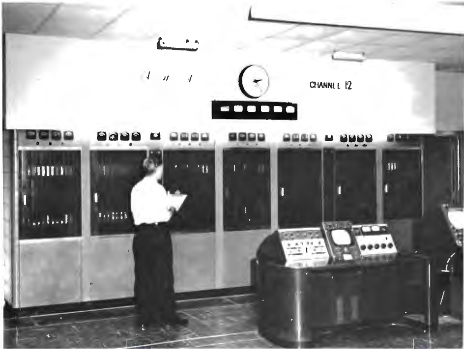
FIG. 24. Type TT-50AH 50-KW TV Transmitter is located in master control room, along with the video control desk and master control switching. It feeds a TF-12BH antenna located behind the studio building on a 922-foot Ideco Tower. The overall height is 996 feet above ground.
