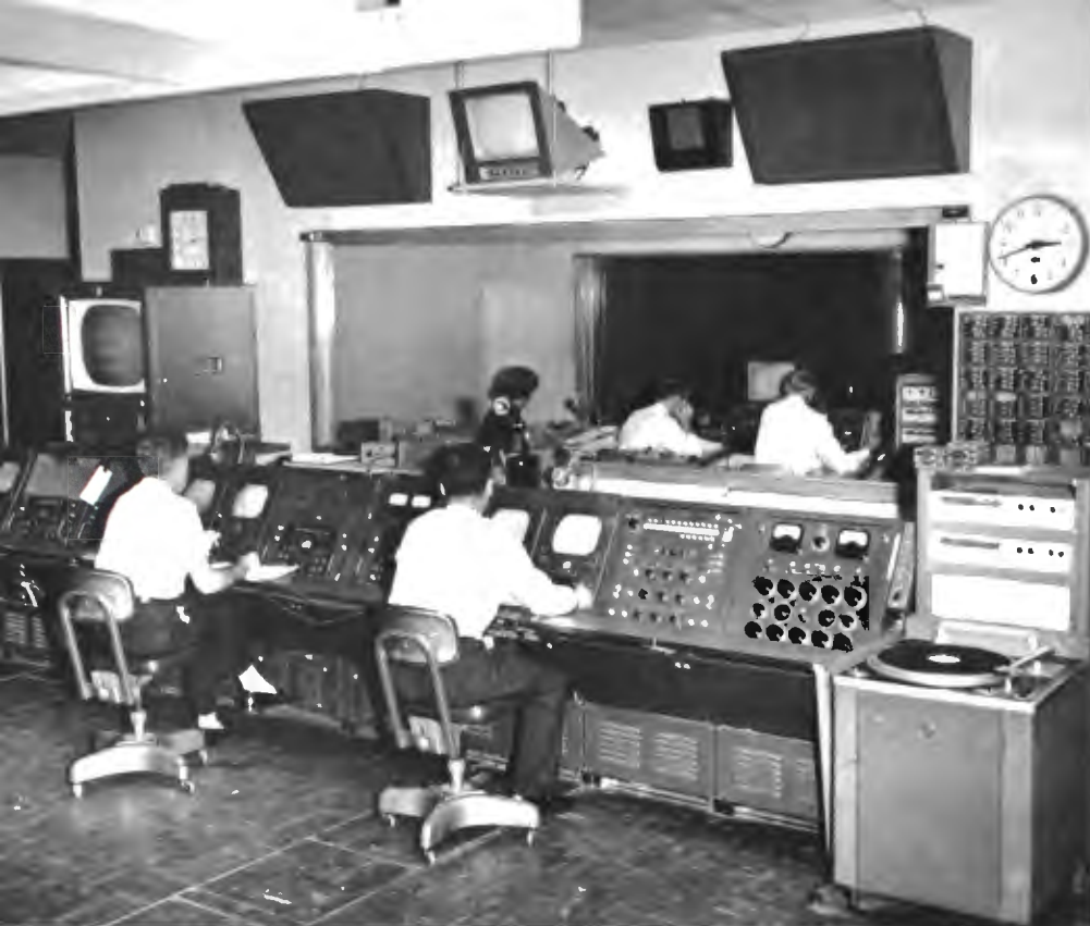
FIG. 21. In background is Control Room "A". Foreground (L. to R.): TK-11 controls; TK-41 color camera controls; TK-26 film color controls; master switchable monitor; master video switching panel; master audio switching panel; cartridge audio tape and RCA turntable.
