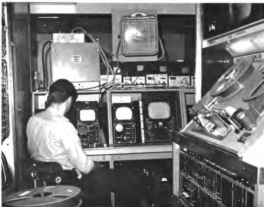
FIG. 25. TV Tape and transmission area in main mobile unit. Video patch, sync, and distribution amplifiers are located here.
