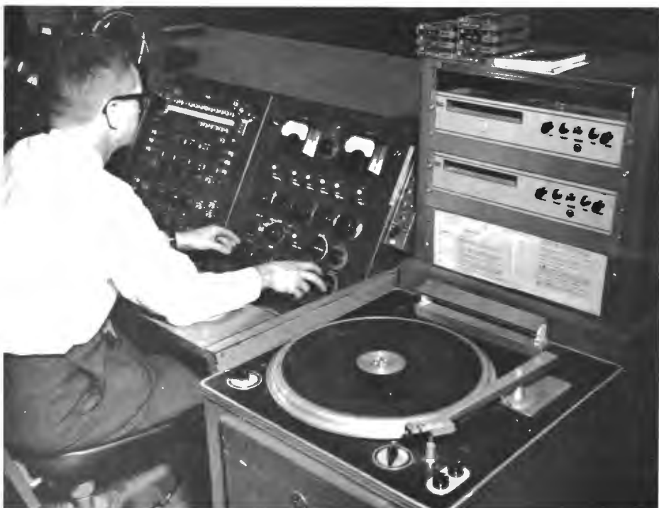
FIG. 22. Master Control Switching. Left panel contains video switching, stab amp controls, and remote start and stop switching for tape and projection equipment. Next panel contains audio program and monitoring equipment. Audio switching is normally interlocked with video, but an interlock defeat switch can lock any program source either in or out. Master Control can handle the air operation while other facilities are being used for TV taping or studio rehearsals.
