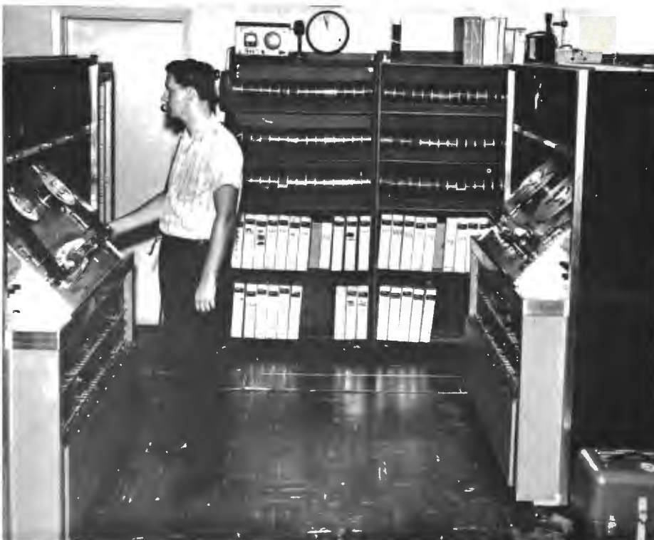
FIG. 18. TV Tape Room is located next to Projection and Master Control. Contains two RCA TR-22 TV tape recorders, with transistorized color modules. (A third TR-22 is installed in WFGA-TV mobile unit.) Recorders have remote start in Control "A", Projection, and Master Control.
